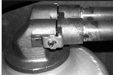
Figure 23-1: Copper tubing soldered to water softener head
