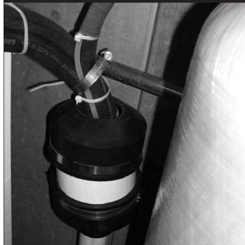
Figure 23-3: Water softener and RO rejection water hoses connected to drain cup
